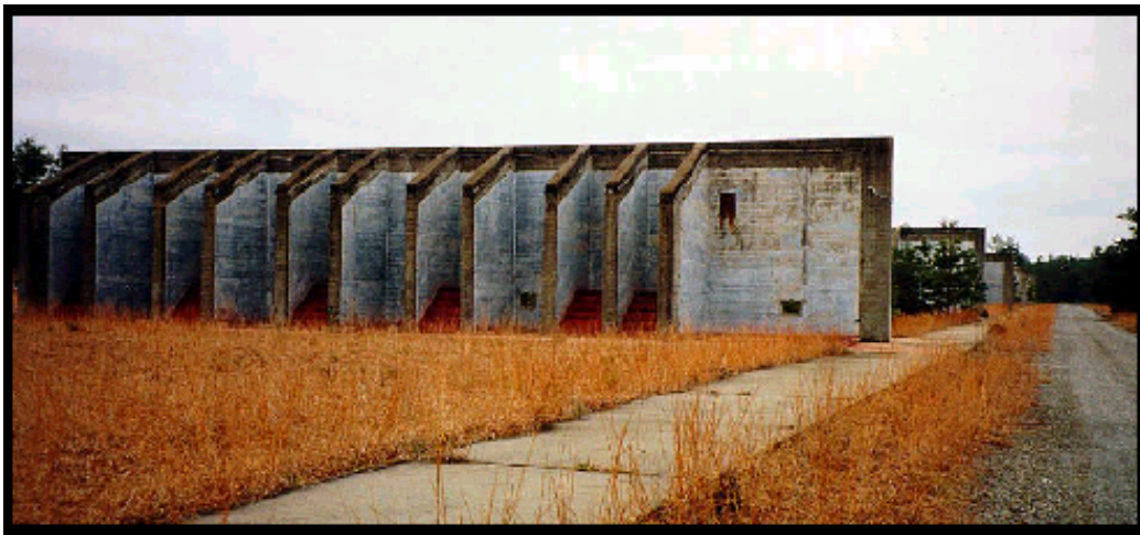
IGNITER ASSEMBLY AREA
